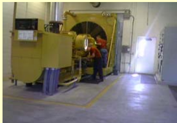
Trussville WWTP: Employees perform preventative maintenance on a generator
